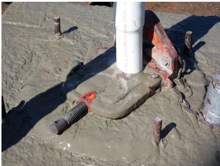
Figure 1. A cement and bentonite clay mixture around the well casing keeps surface water and pollutants from reaching the water supply.
